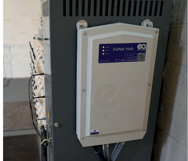
Figure 1: VisNet® Hub installed in a substation in the Marches region.
