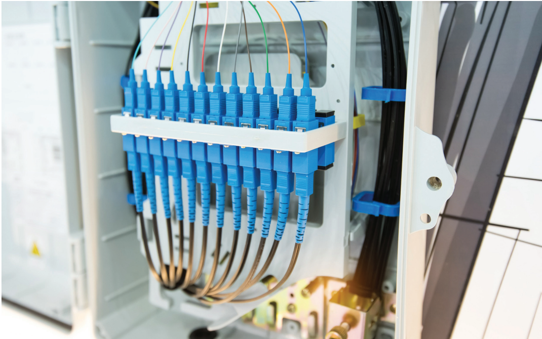
Figure 3: Fiber Patch Panel
