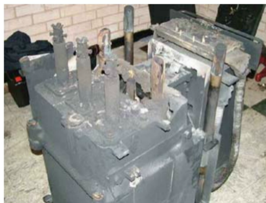
A failed oil filled circuit breaker, shipped to our laboratories for investigation
