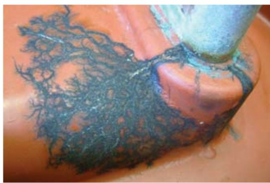
PD activity on a cast resin monobloc, caused by a poor substation environment
