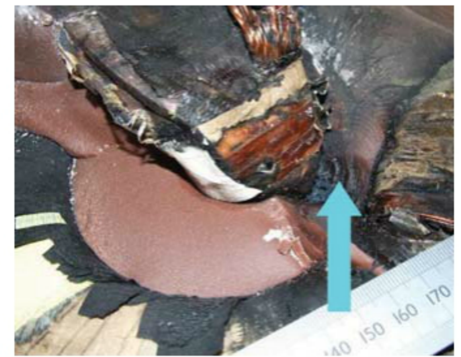
Foreign body in failed CT winding
