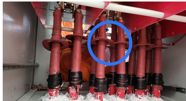
Figure 3: Location where PD was detected.
