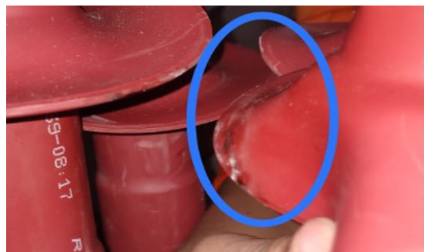
Figure 4: Physical signs of PD on the anti-tracking sheds.
