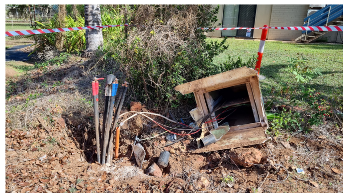
Figure 3. LV pillar crash site
