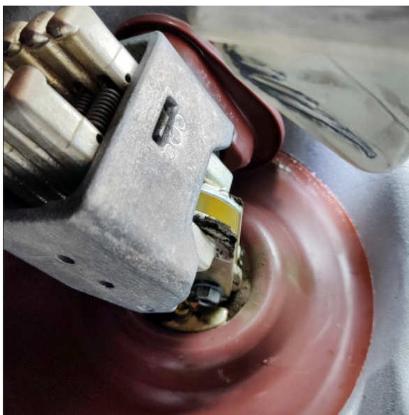
Figure 1: 33kV switch contact which was the source of the PD.
