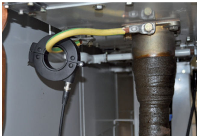
Figure 2 RFCTs installed on the earth conductor of single-core cables.
