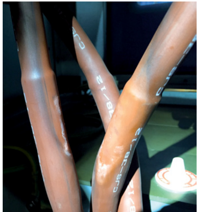
Figure 1 Partial discharge caused by incorrect installation found on a cable termination using non-intrusive PD 'UltraTEV' instrument
