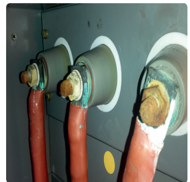
Evidence of PD at site brought to light by UltraTEV Survey
