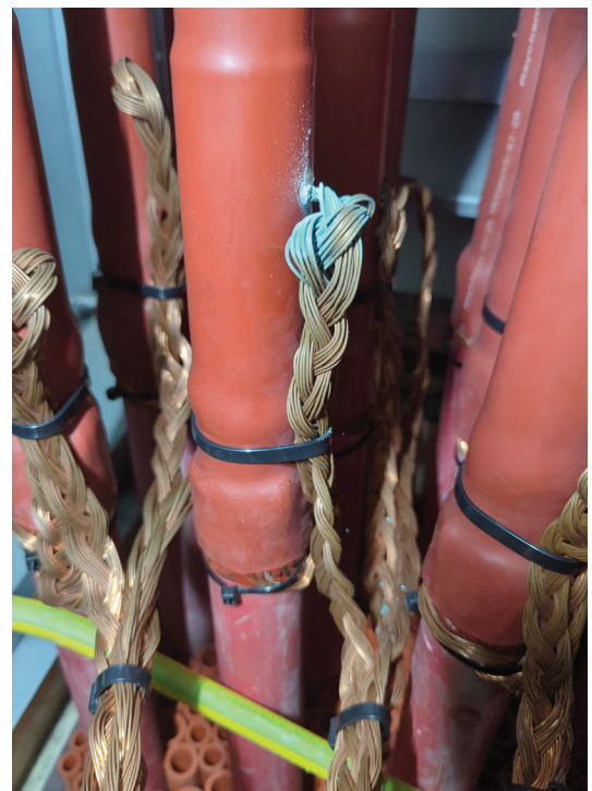
Figure 6b: Geometrically Induced PD on Braided Grounds
