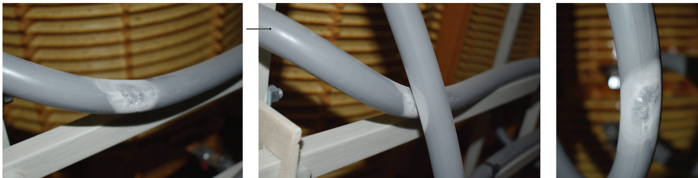
Figure 3b: PD Due to Physically Touching Cables
