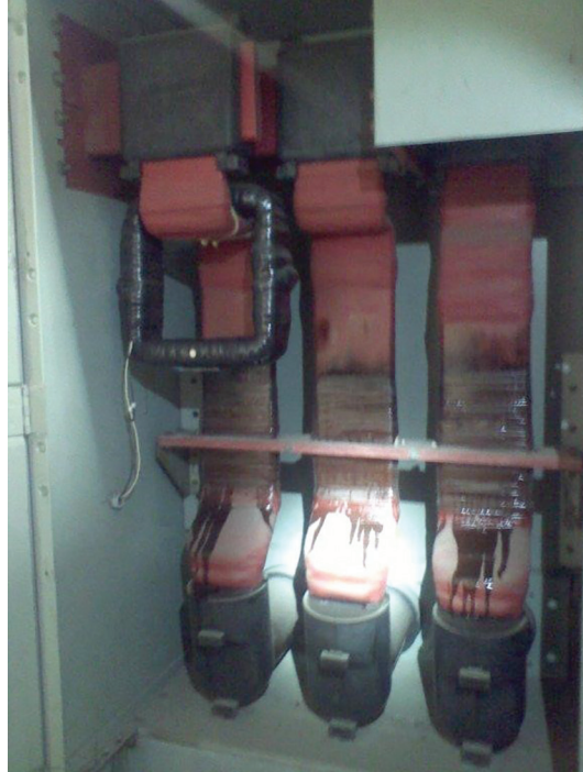
Figure 8a: Busbar Bracket with PD Damage
