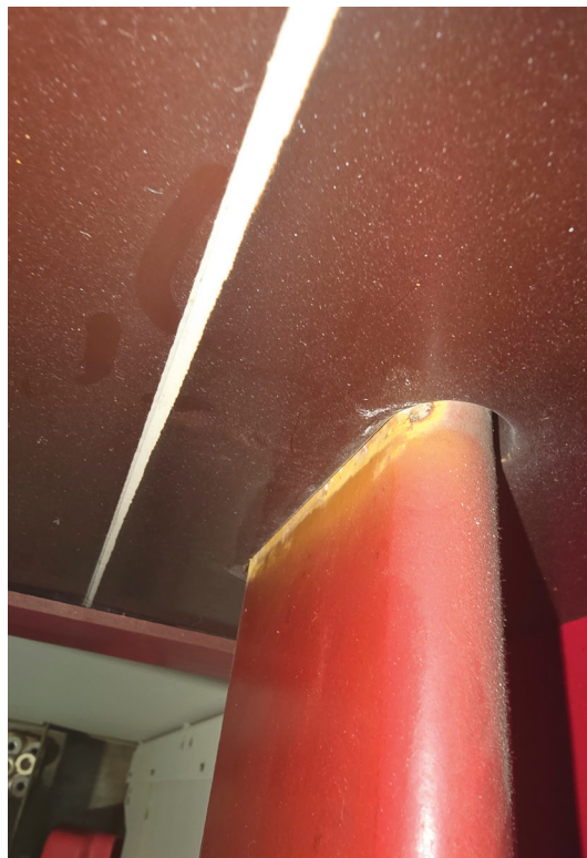
Figure 2: Bus Bar Going through Oversized Hole in Panel
