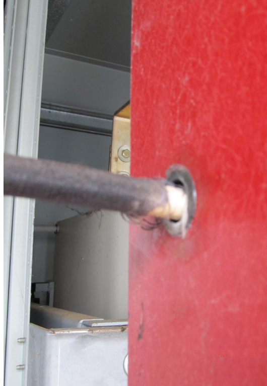
Figure 1: Air gap in Grommet Causing PD
