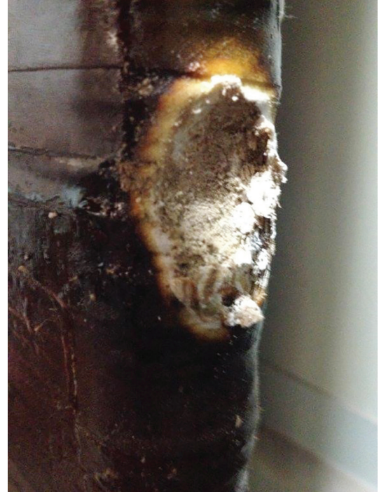
Figure 8b: Closeup of PD Damage
