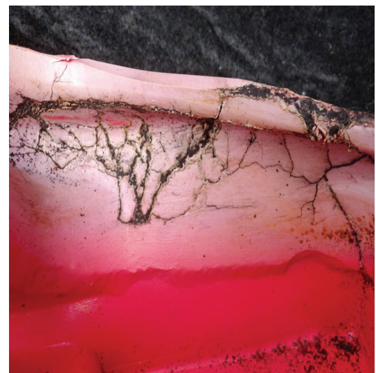
Figure 3a: Boot Installed with Insufficient Air Gap and Resulting PD Damage
