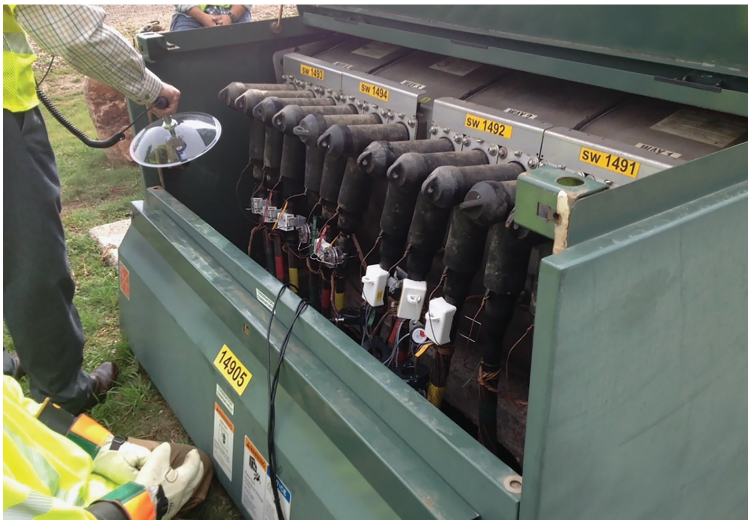
Using a Parabolic Ultrasonic Selector on Pad-Mount Cable Terminations
