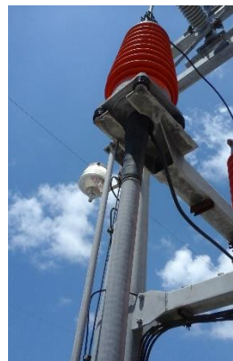
Cable termination in 69KV switchyard
