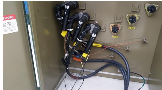
Cable termination in metal-clad switchgear
