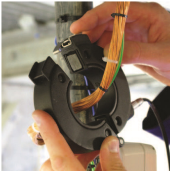
Split core HFCT applied to HV cable earthed screen wires
