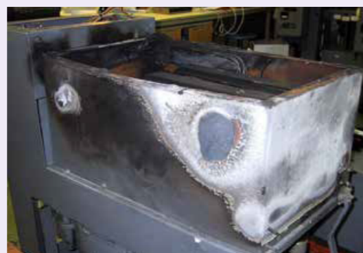
Explosion in 3.3kV circuit breaker.
