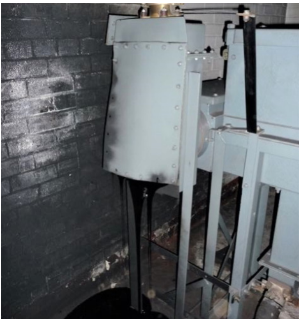
Figure 1 Failed bitumen filled cable box
