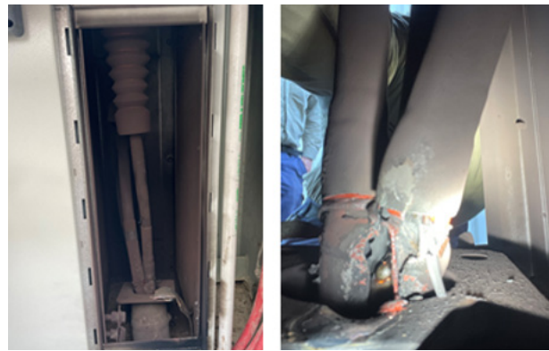
Figure 4 11kV RMU Termination Failure
