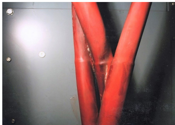
Figure 2 Phase to phase PD caused by poor installation
