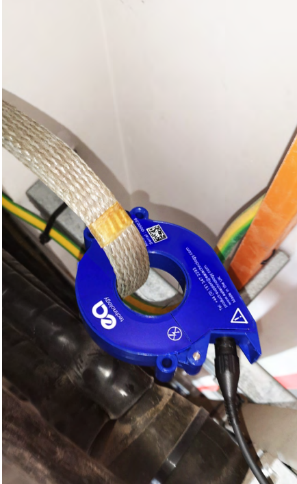
Figure 4: HFCT on earth braid of HV cable
