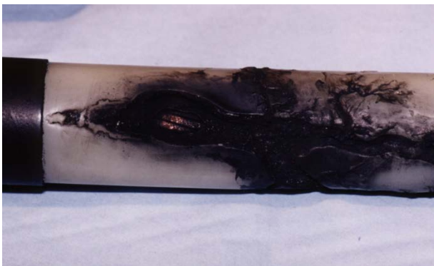
Damage from flashover to screen
