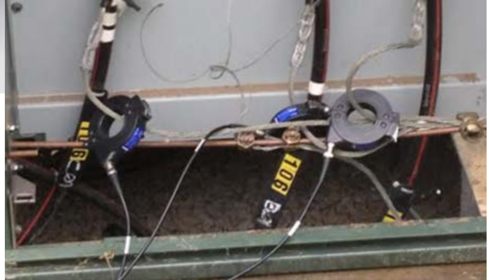
RFCT Installed on Ground Straps
