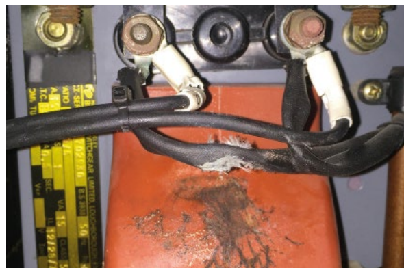
Figure 1: Partial discharge identified.
